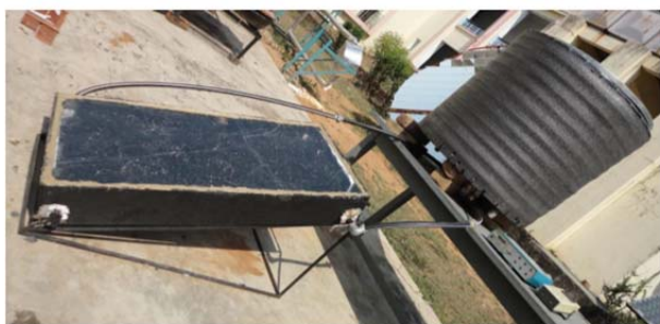
Fig. 3.2a: Working model of the flat plate solar water heater
